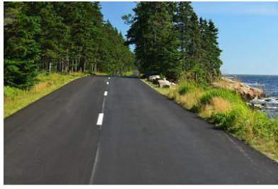
Freshly paved highway traveling along the Schoodic Bay in northern Maine, by Jorge Moro, Shutterstock .
